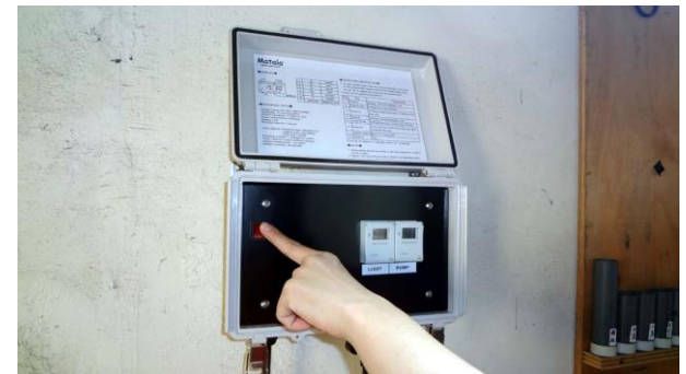
9, Power on and start the fountain system
