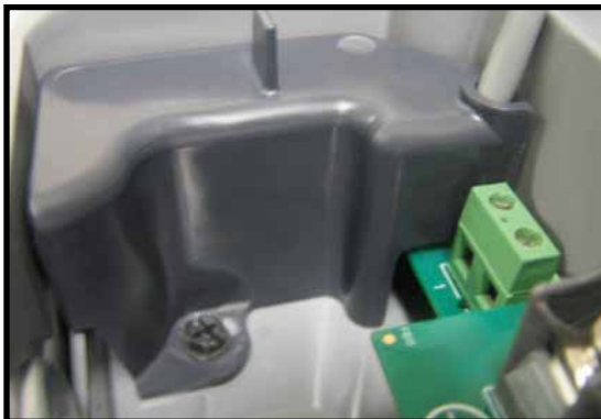
Figure 15: Plastic Cover Installed In Terminal Box
